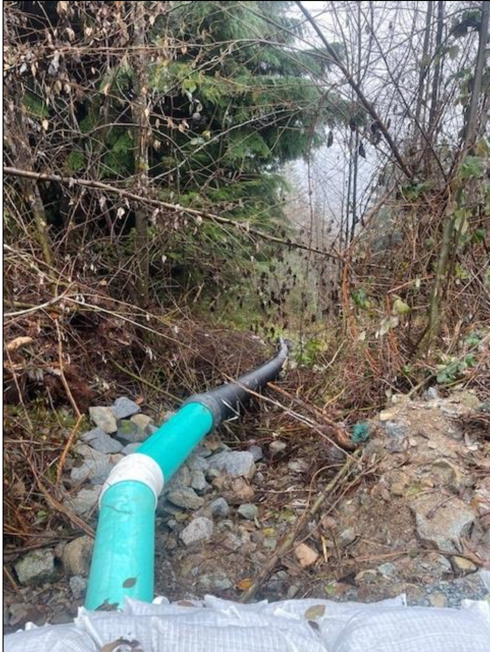
Photo 8: Minor Drainage System # 2, stormwater drainage pipe at south extent of asphalt paved Ridge Mountain Drive, collecting drainage from the swale shown in Photo 7, looking downslope/west (December 11, 2023)
