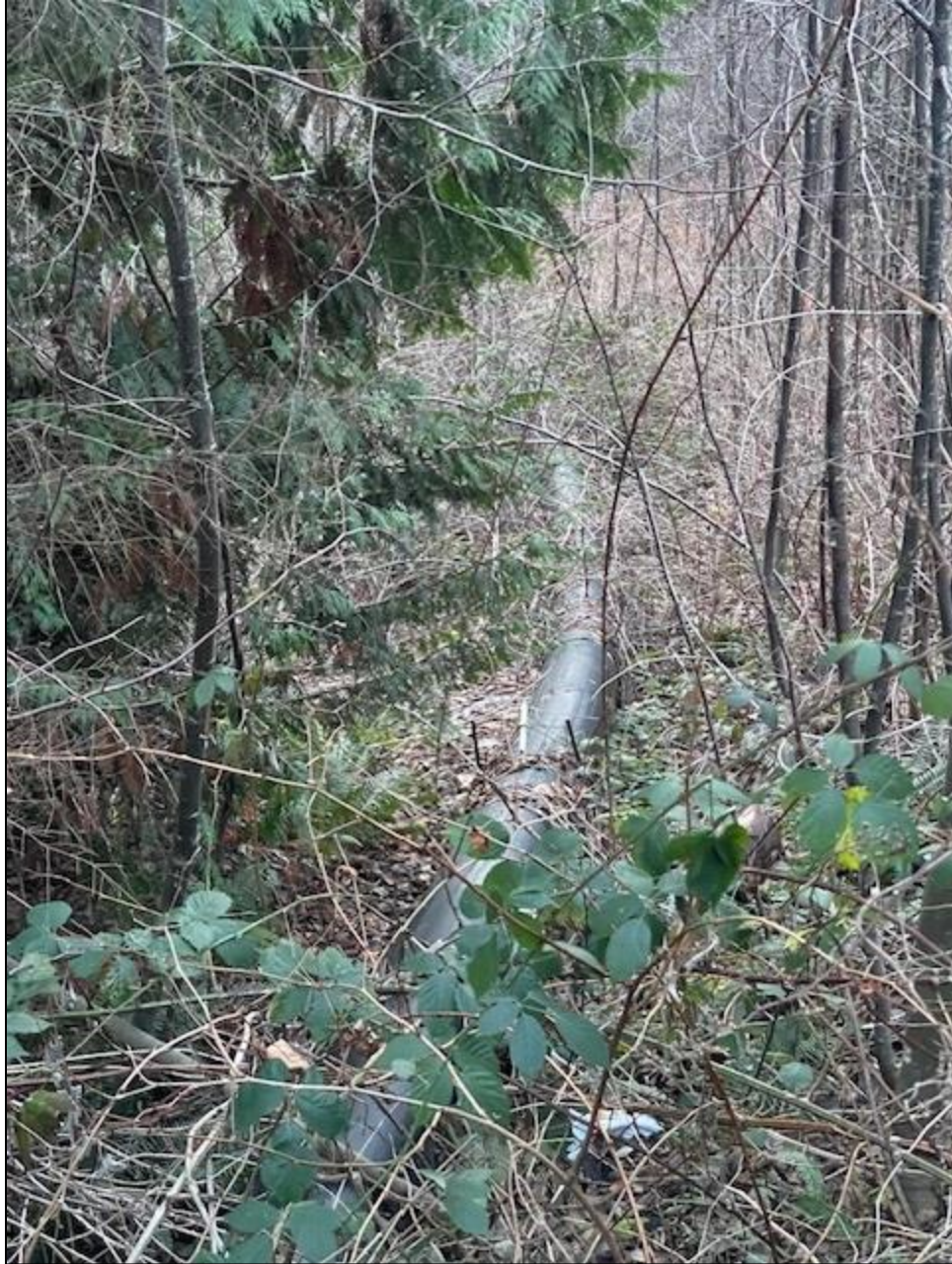
Photo 21: Minor Drainage System #2, stormwater drainage pipe at west side of North Charlotte Drive extension (December 13, 2023)
