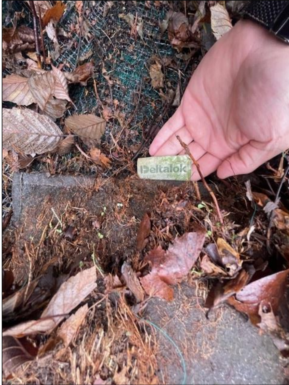
Photo 14: Downslope drainage swale at southern portion of TREZ development showing Deltalok™ Geo-Modular Bags (December 13, 2023)
